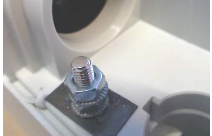
Protective earth, metal pin
