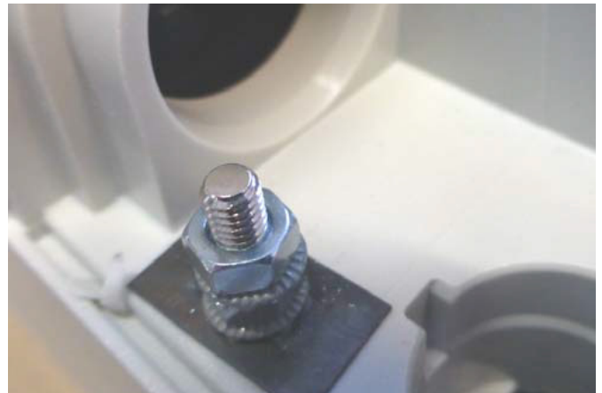
Protective earth, metal pin
